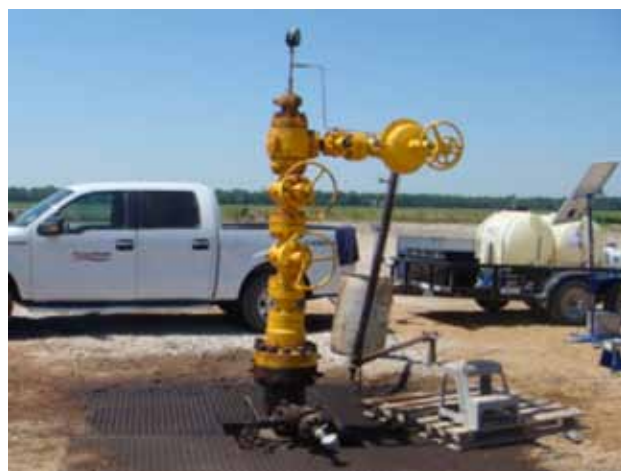
Deshotels 20H No. 1 Production Well Head
